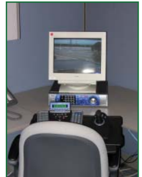
Additional computer work-space and camera controls with recording capabilities.
