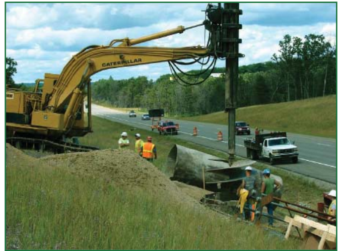
DMS foundation being installed on southbound I-75 in Crawford County. photograph by Steve Zaglaniczny, July 12, 2007
