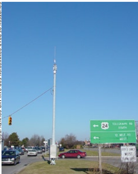
A test-bed installation at Telegraph and 12 Mile Roads in Oakland County.
